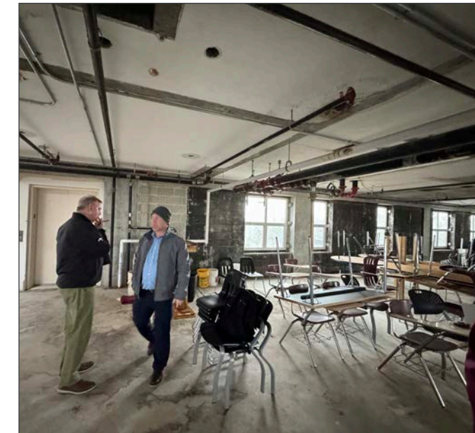
4th floor before: Concrete slab and column grid, the room’s working bones
